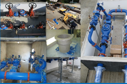
L-R: Backflow/Meter Station, Chambers Arriving for Assembly, PRV Station in Chamber, PRV Station in Concrete Building, Pipe Spool Ready for Paint and Galvanized Steel Pipe Stands
