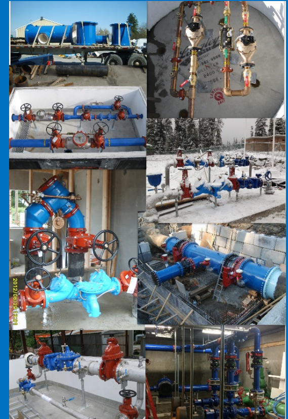
L-R: Spools Ready for Delivery, Meter Station in Manhole Barrel, Backflow Chamber, Aboveground PRV Station (Kiosk not installed yet), Backflow Station in Building, Large Diameter Piping with Valves, Stainless Steel PRV Station, Pump Station Retrofit
