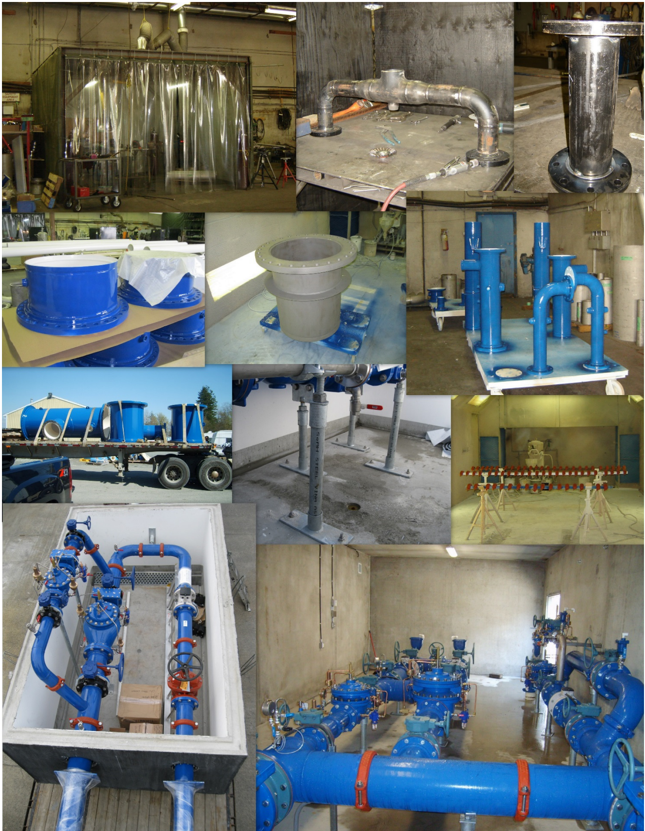
L-R: Stainless Steel Fabrication Booth, Pipe Spool in Various Stages of Fabrication, In house Pipe Spool Coating, Stock Galvanized Steel Pipe Stands, Victaulic Epoxy Coating, PRV Station in Chamber, PRV Station in Concrete Building
