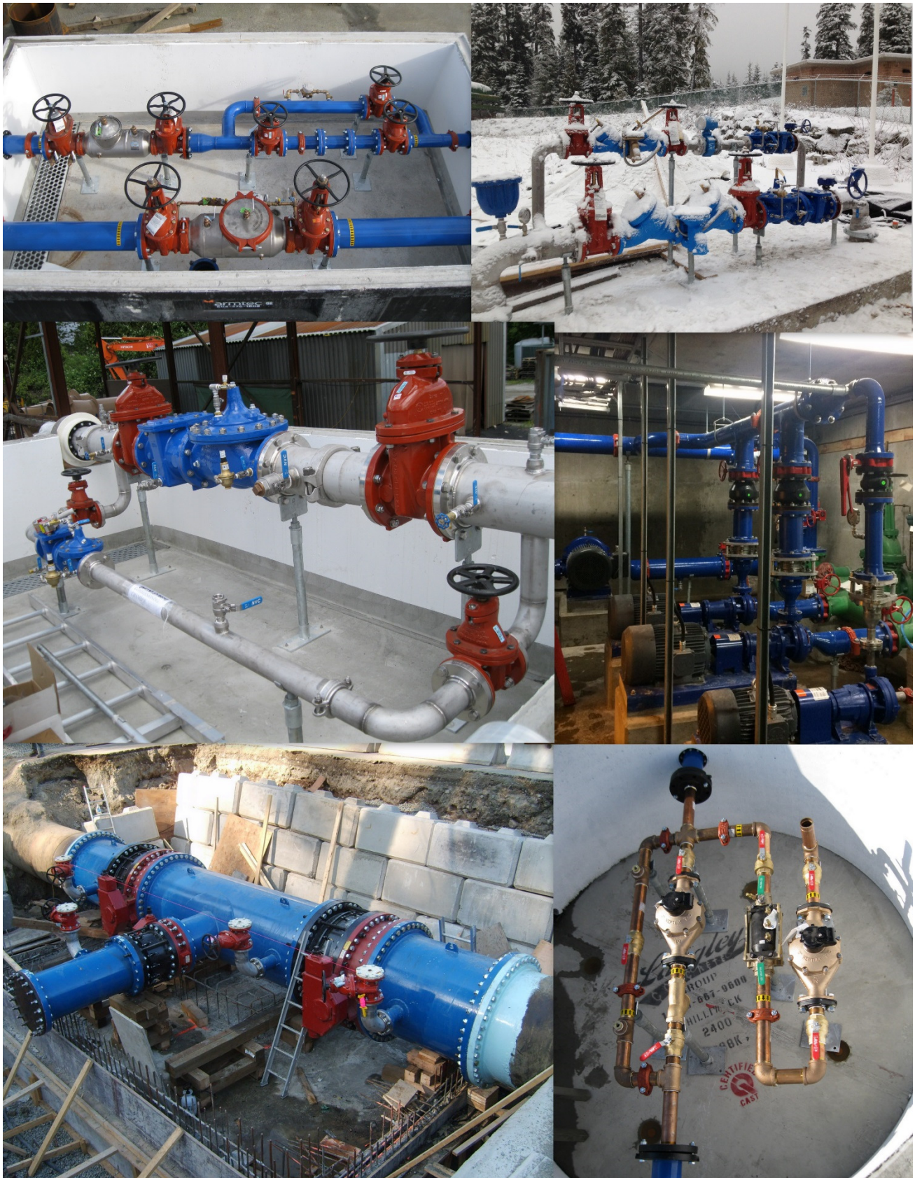
Backflow Chamber, Aboveground PRV Station (Kiosk not Shown), Stainless Steel PRV Station in Chamber, Pump Station Retrofit, Water Main Replacement, Meter Station in Manhole
